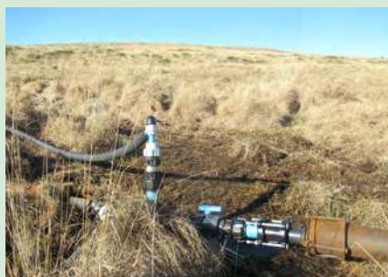
The new pipework
