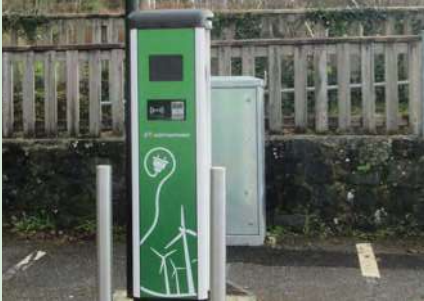
The new recharging point
