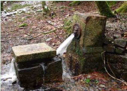
The damaged fountain
